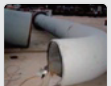
Loob ng welded pipe
