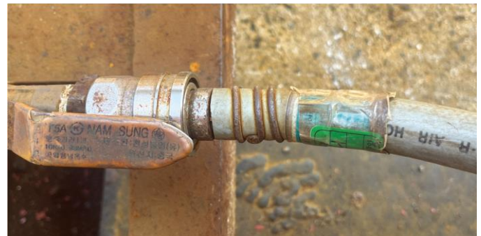
Failure to use clamps
