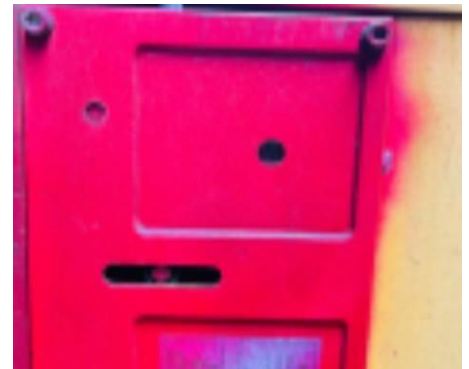
Check the operating status of the overload protection device.
