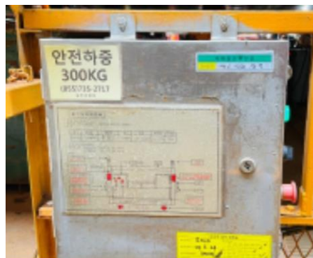
Check for any irregularities in the control panel instruments.
