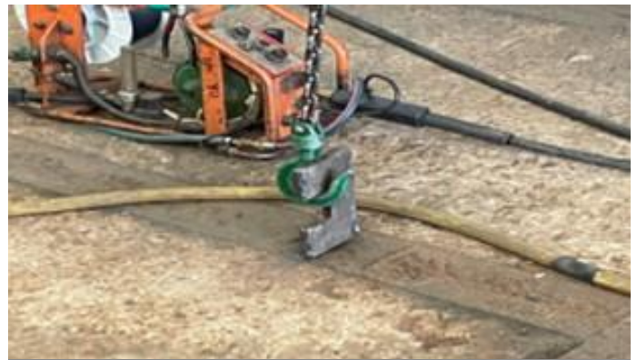
Attaching to a structure at risk of the hook detaching
