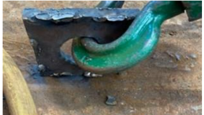
Attaching to a lug with insufficient welding
